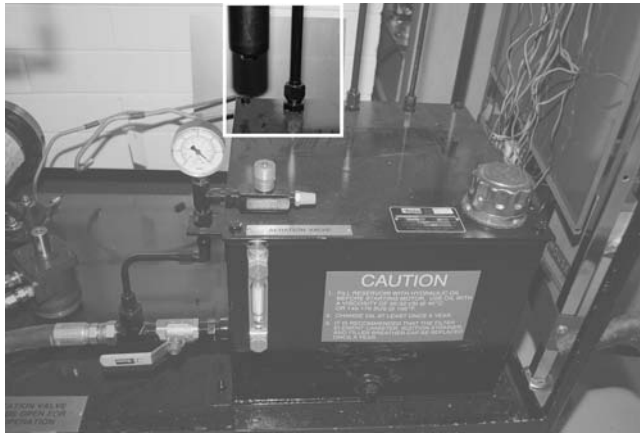
Figure 2-51 In this system, the highlighted return line is connected to the reservoir with a lightweight and relatively weak compression fitting. Rigid piping like this is typically only used in locations where the piping and reservoir can both be rigidly mounted to a framework or panel.
