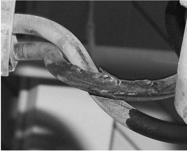
Figure 2-45 Many hoses in a fluid power system are sheathed to protect them from rubbing on the mechanical components of the equipment. Improper maintenance or failure to protect the hoses from being chafed by moving components can damage the hose and possibly cause system contamination and massive leaks.
