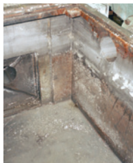
Corrosion in the reservoir
