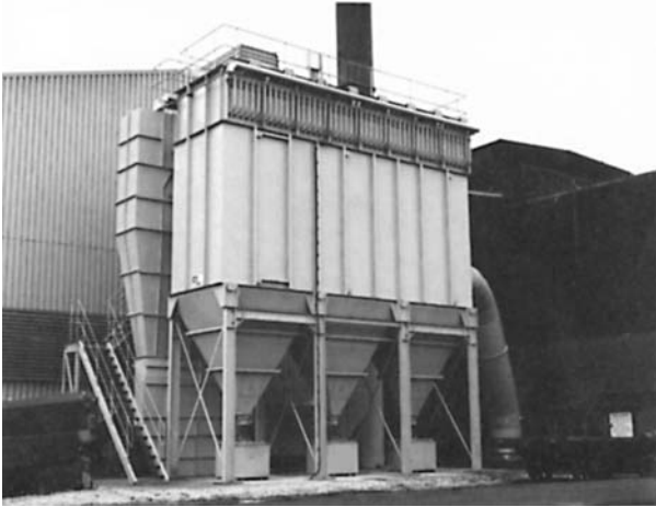
Figure 6.25 Fabric filter with vertical elements
