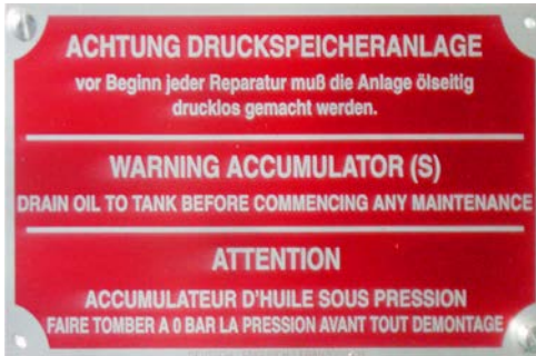
Fig. 21 Warning note on accumulator system
